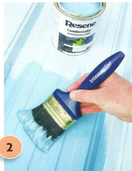
2 Apply two coats of Resene Norwester to both sides of the panel (if painting it), allowing two hours for each coat to dry.
