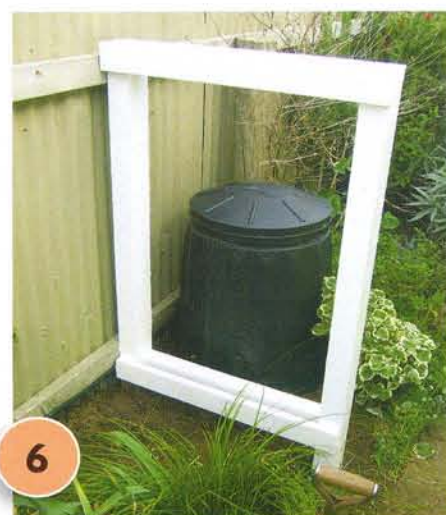
6 On the right-facing side, nail the two remaining cut lengths of 100mm x 50mm across the top and bottom of the frame (drill pilot holes first). Apply one coat of Resene Quick Dry to the entire frame, allowing one hour to dry.
