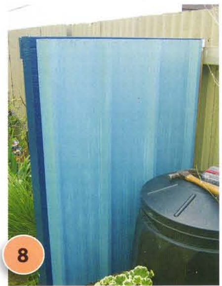
8 Fix the painted panel to the back of the frame, nailing with 40mm flathead nails along the top and bottom edges. Spot prime and paint the nail heads.
