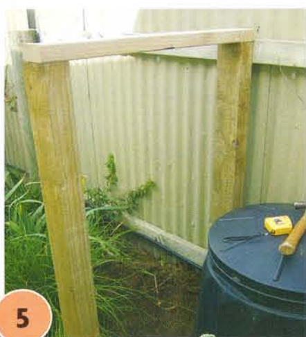
5 Attach a longer cut length of 100mm x 50mm timber across the tops of the posts with 100mm nails (drill pilot holes first). Fix the short length of 100mm x 50mm between the posts about 1250mm from the top edge by 'skew' nailing it at an angle (drill pilot holes first).
