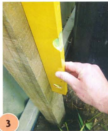
3 Dig a hole about 500mm deep and position the first fencepost. Use a spirit level to ensure the post is upright and fill in the soil around the base of the post, compacting the soil as you go.
