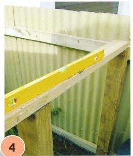
4 Repeat step 3 and position the second fencepost 720mm away from the first. Rest an offcut of wood across the tops of both posts and use a spirit level to ensure both posts are the same height.
