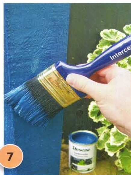
7 Apply two coats of Resene Prussian Blue to the entire frame, allowing two hours for each coat to dry.
