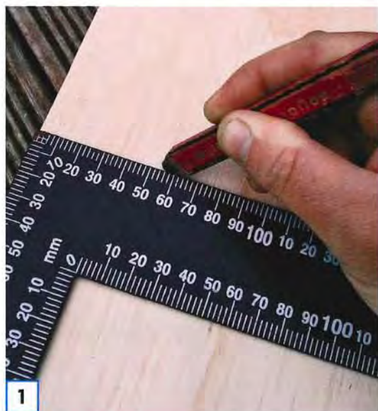
1 Measure and mark the pieces of plywood to the dimensions listed above.
