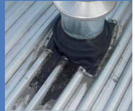
Poorly fitted penetration causing ponding and debris build up.
