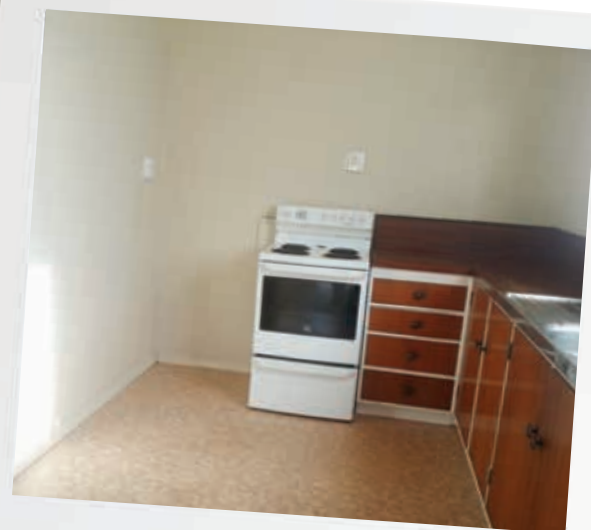
Kitchen before: Tenant, Tom, removed the kitchen cabinets, stove and sink before the fitout.
