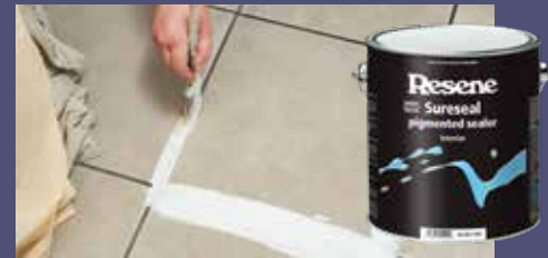
2: Apply one coat of Resene Waterborne Sureseal to the tiles and grout and leave it to dry. Use a cutting in brush for the edges and grout, then a roller for the tiles.
