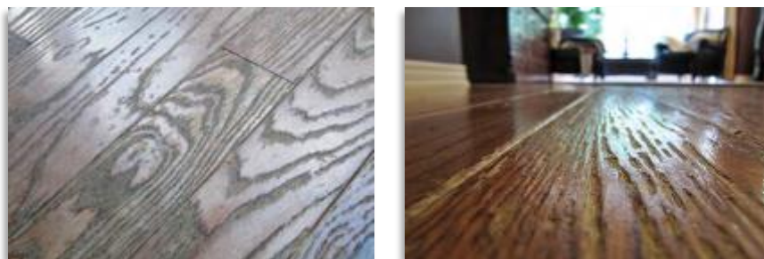
A prefinished timber floor damaged by repeated use of a steam mop cleaner.
