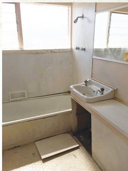
ABOVE The old bathroom needed to be completely replaced. RIGHT A strong back deck was installed to replace the substandard existing one.
